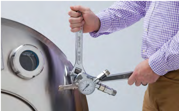
FIGURE 11: SECURING THE PRESSURE SAFETY VALVE
