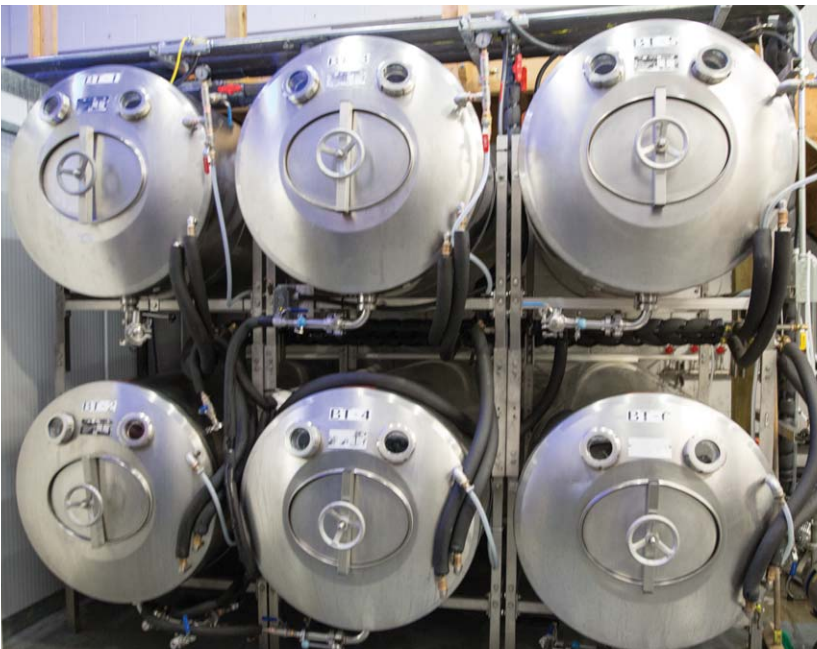
Serving beer tanks in use in Kitchener, Ontario.
